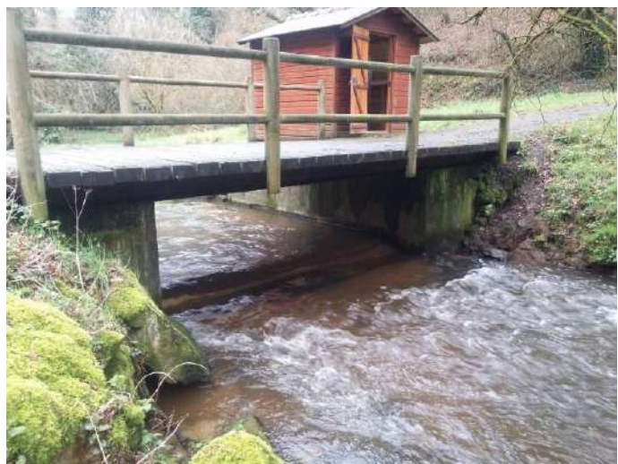
Station J1524010 La Maudouve
